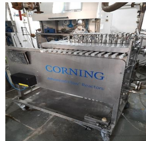
Corning G4 Reactor (Plant Set-up)
