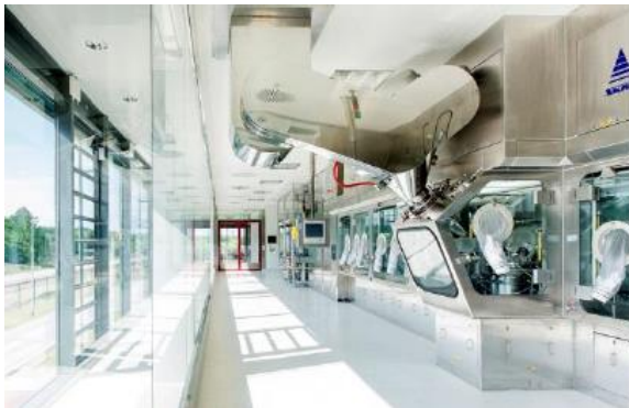
Isolators for production filling lines
